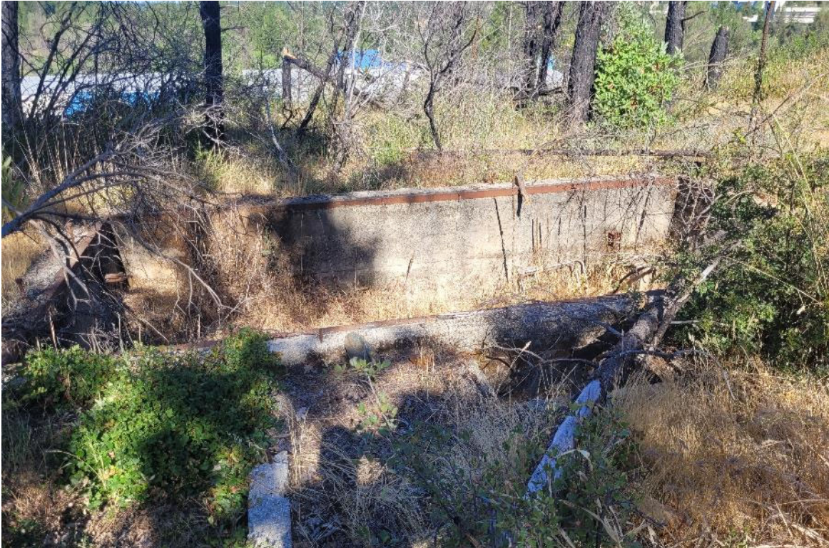
Photo 11 – View to the west of a concrete basin, possibly on adjacent property, near the northwestern site boundary.
