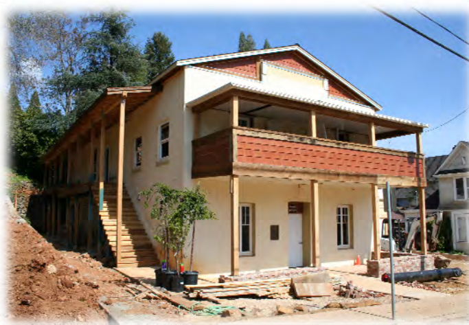
Rehabilitation involving reuse of historic fabric and replacement materials that match the building's original design and fabric.
